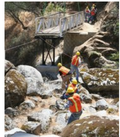
Volunteers maneuver sections of a bridge into place at Big Sandy Creek. "The civilians hadn't done anything like this before. Honestly, we hadn't either," said National Guard Lt. Col. Mark Van Dyke, who piloted the helicopter that hauled the bridge sections. California Department of Parks and Recreation
